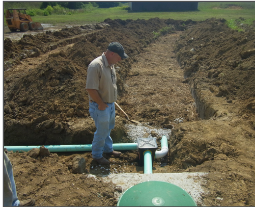
One of many septic replacements performed under the previous Bacon Creek 319 grant. The new grant cycle will enable many more septic fixes that help clean up Bacon Creek.
