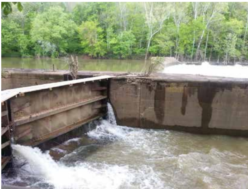
This photo by Judy Petersen captures the hazards created by the failing Green River Lock and Dam 6. The resulting ledge, sieves, and strainers can be deadly obstacles for unsuspecting boaters. These threats will persist and worsen in some instances if these old structures remain.
