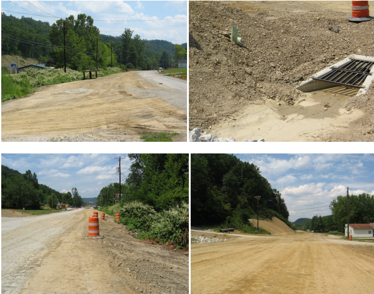
Figure 3.14: Sample of images taken during KY 519 construction, which show a complete absence of the erosion prevention and sediment controls required by state contracts.
